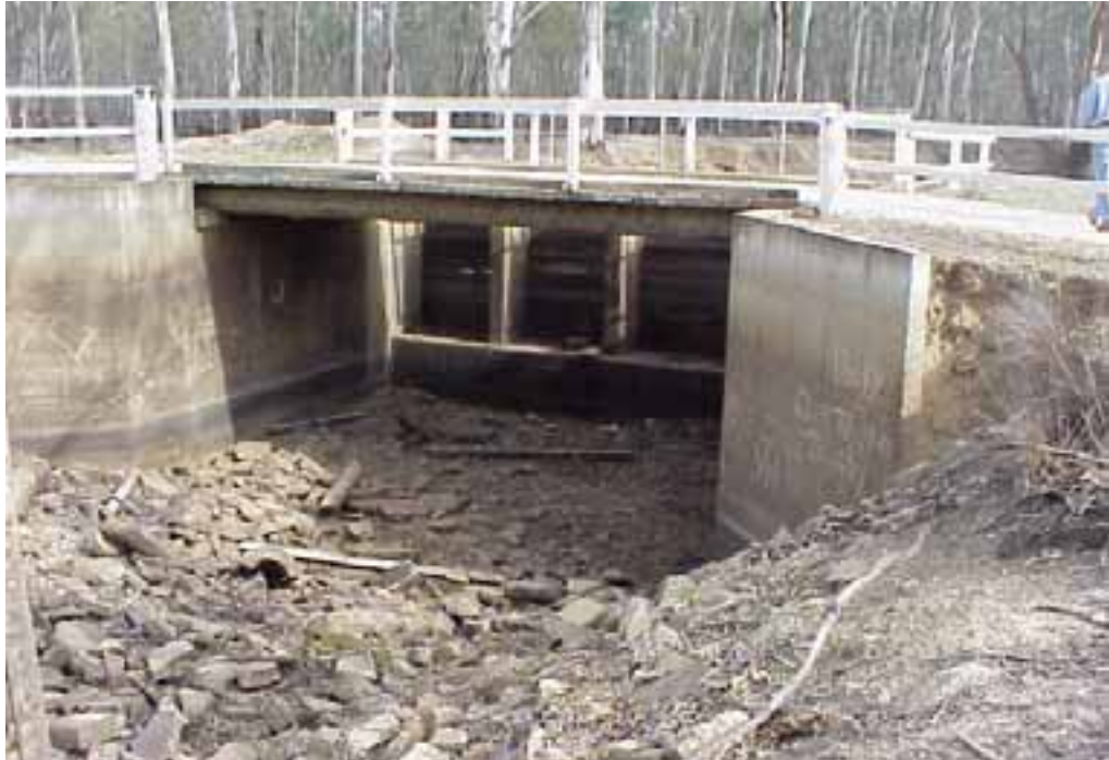
Figure 3.7 – Shillinglaws Regulator when closed (photograph: supplied by Emer Campbell, North Central CMA)
